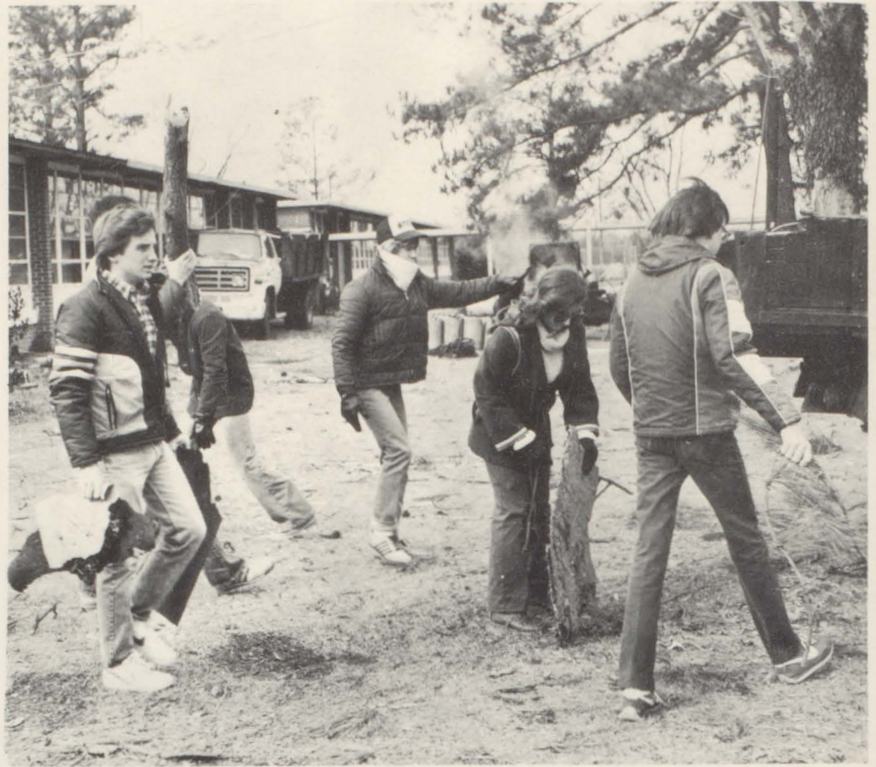
Members helped clean up the Middle School after the tornado.
