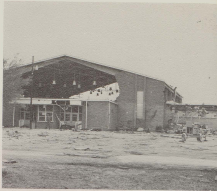
The gymnasium was virtually blown apart from the pressure.
